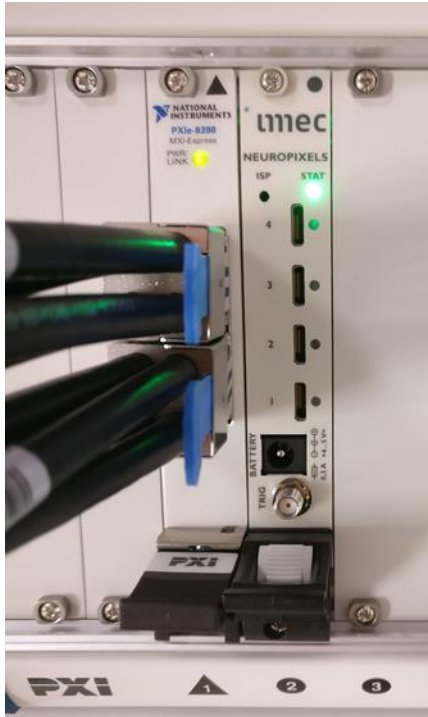
Figure 24: Global status LED of the PXIe acquisition module switching from red to green after correct installation.
